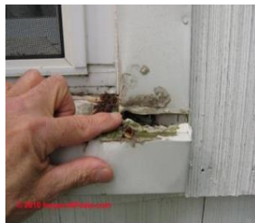
Improper Installation may cause unnecessary damage to the building
