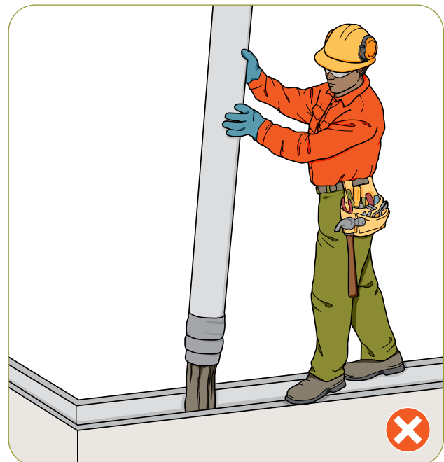
Don't walk on the top of formwork.
